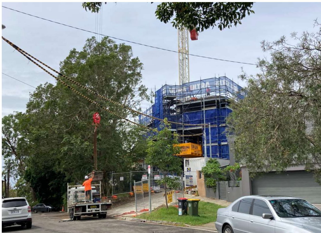
Figure 7: Residential flat building under construction at 21-23 Riddell Street, viewed from the street frontage.
